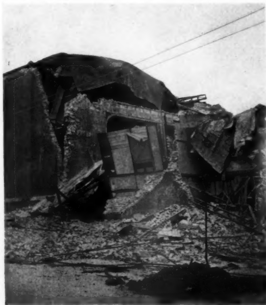
FIG. 8. TYPICAL DESTRUCTION OF BRICKWORK
